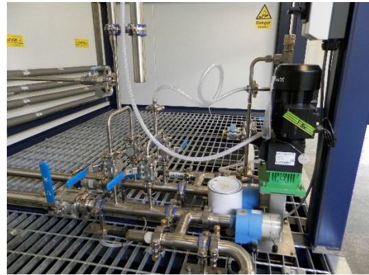
IBC Dosing Station E/2/1000 Internals
