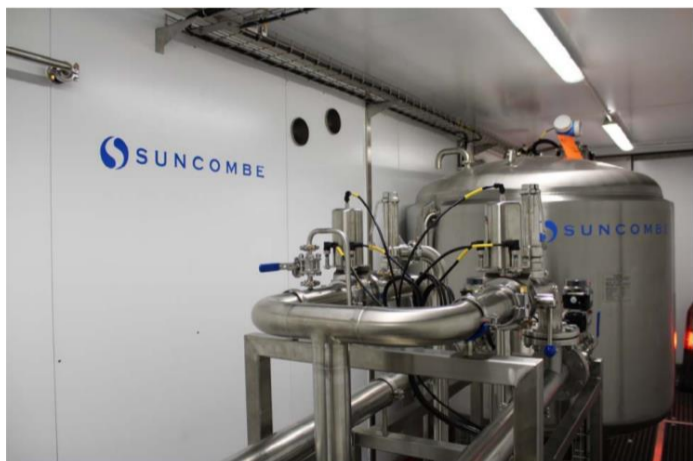
Utility Container Internals
