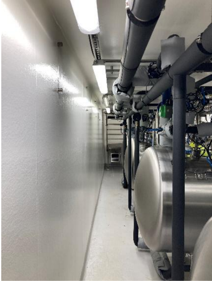
Treatment Hall Internals
